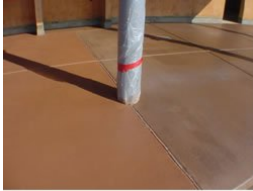
Photo: Batch to batch quality and quantity of ingredients should be closely monitored and controlled to avoid such visible color difference. Source: www.concretenetwork.com
